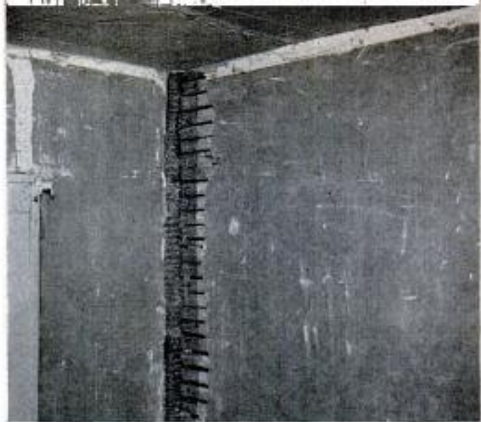
Old plaster has been removed from cracked area at corner of room. Expanded metal lath is nailed in corner and area is replastered along with ceiling
